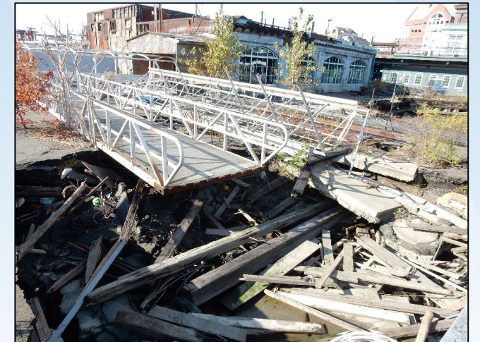
Immigration & Pullman Building (background) being reconstructed to house a storm resilient substation
